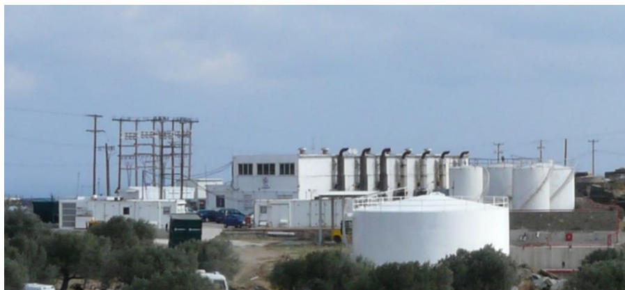
Figure 5 : PPC's diesel power plant in Plakoto, Sifnos with exhaust pipes of seven fixed gensets (centre), fuel tanks (centre and lower right), two containers with mobile gensets (centre and left) and the 1.5 kV distribution lines (left)
